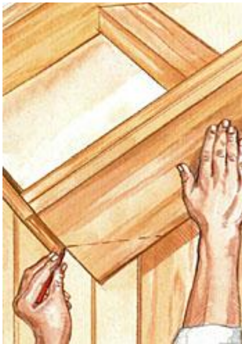
Mark the side fascia so it tapers with a horizontal line that meets the bottom edge of the 1 \times 4 front fascia.
